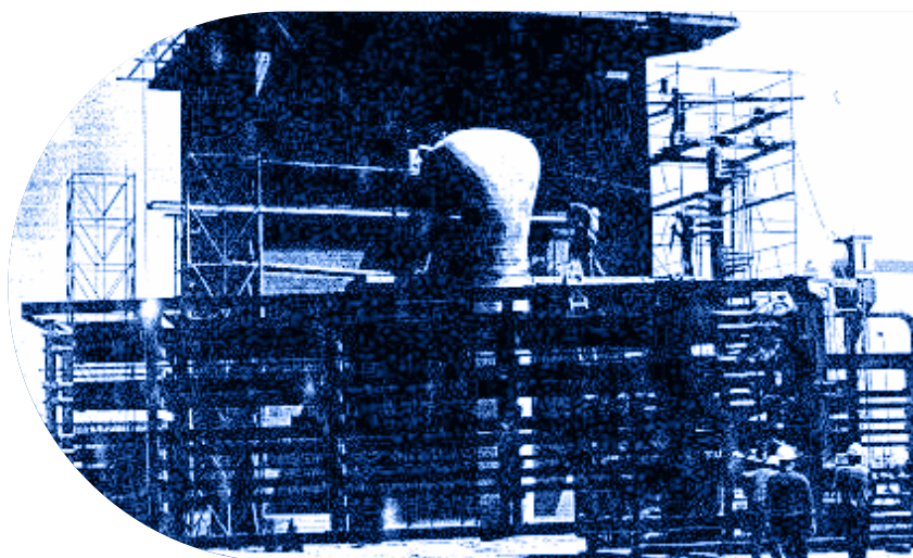
Air Liquide sells 12 vaporizers to LNG import terminals in Spain, Taiwan, South Korea and France
